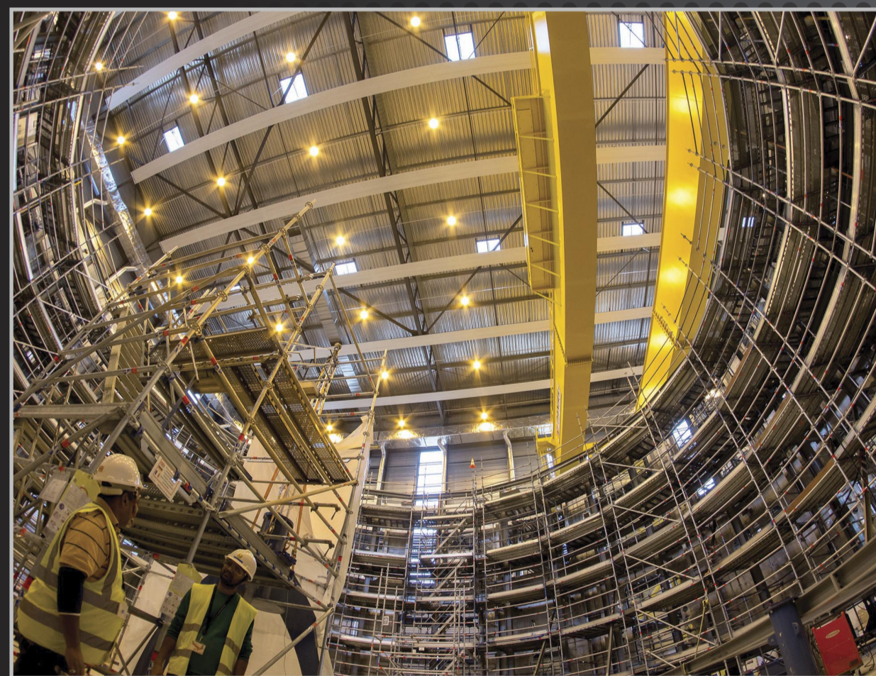
The four main sections of the cryostat are the base (top photo), lower cylinder (pictured), upper cylinder and top lid. In all, 54 steel segments that are manufactured in India and shipped to ITER for on-site assembly in the Cryostat Workshop.
