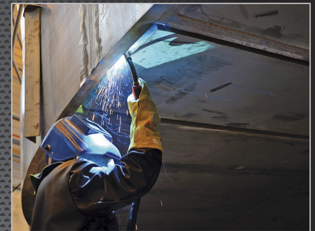
Over one kilometre of welds will be necessary to assemble the segments into sectors in the Cryostat Workshop at ITER. Given the importance of high vacuum in the cryostat, each weld is verified through multiple leak detection techniques.
